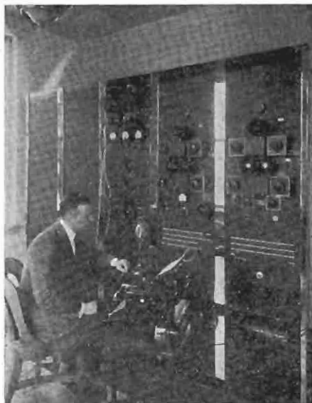
This is the control room apparatus of WEAJ at Bellmore, N. Y. At the left is the oscillograph on which a continuous moving picture of the station output may be observed.
