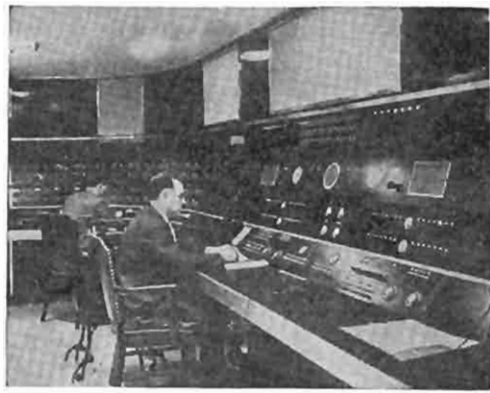
Here we have the "nerve center" of the Red Network—the master control panel of WEAJ in the NBC headquarters in Radio City. Through this exchange, the various studios are connected with the nationwide networks which carry the programs to stations all over the country.
