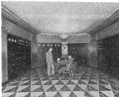
The main transmitter room of WEA. At the left are shown the low power units including modulating and frequency control devices. In the left center is the 50,000-watt power amplifier. In right center is the 20,000-volt high power rectifier. At the right is the power control equipment and dummy antenna system.
